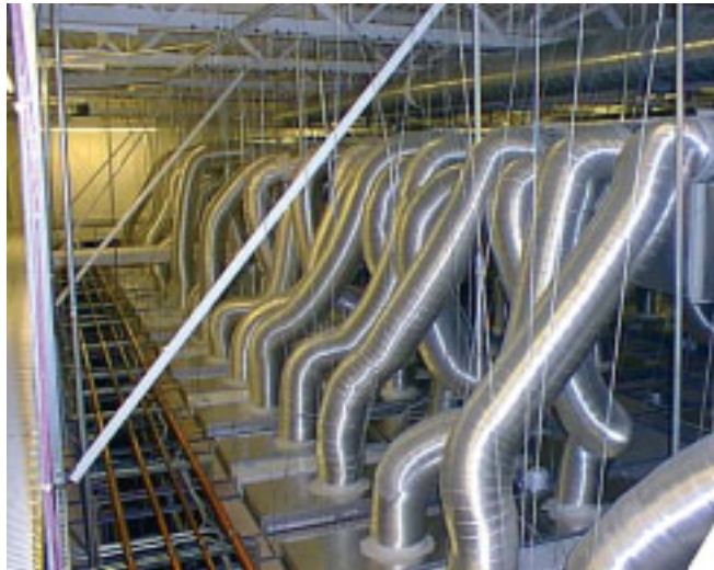
Ducted HEPA filters serving a cleanroom.
