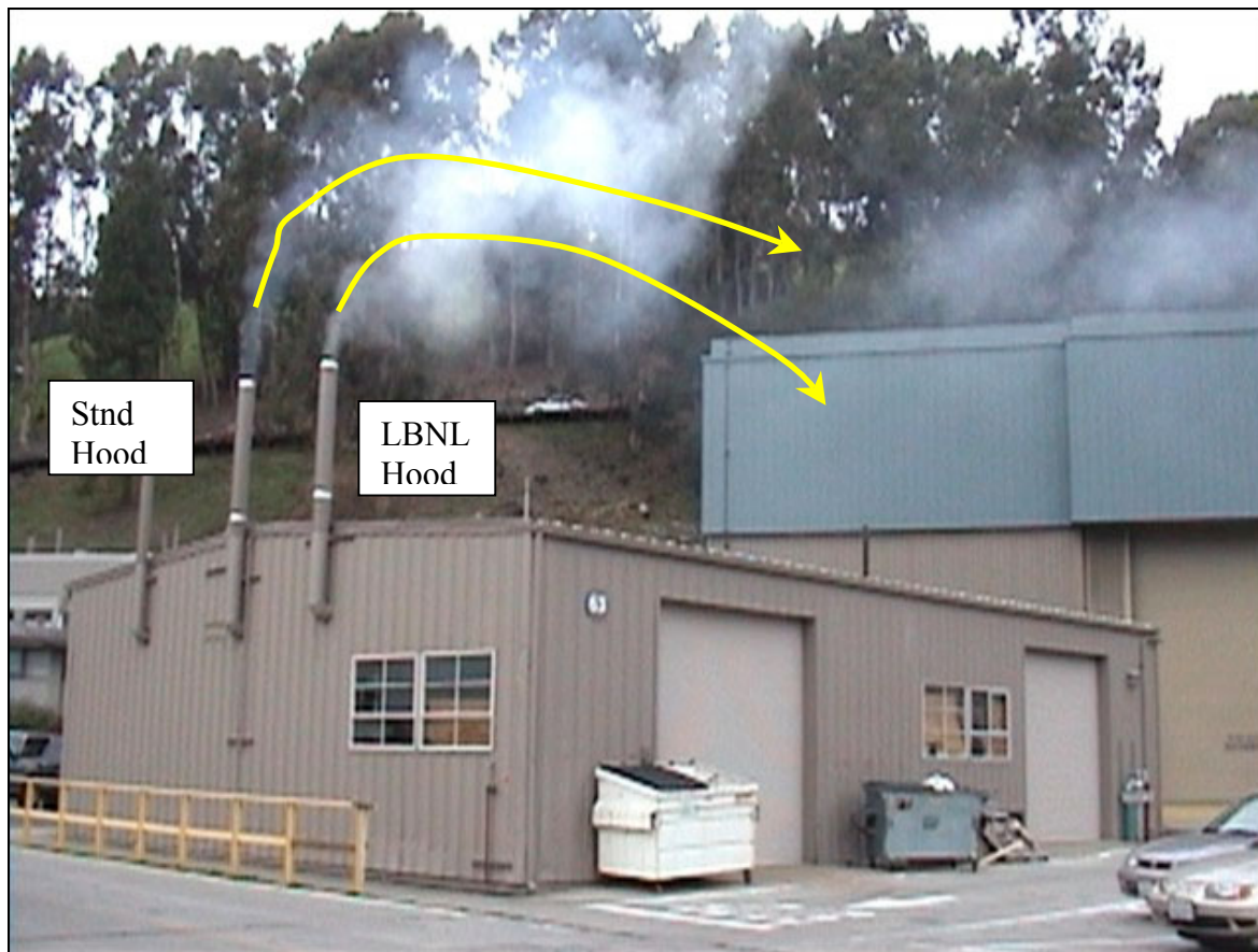
Figure 35 Photo of exhaust discharge from the exhaust stacks serving the LBNL hood and the standard hood.
