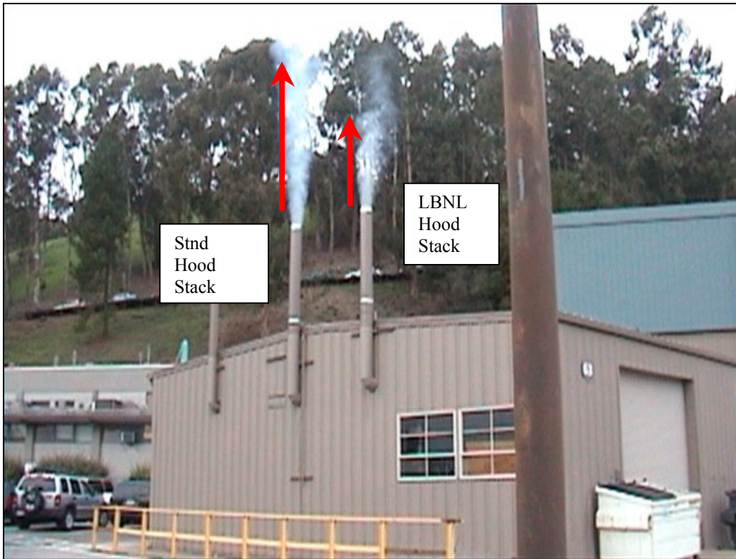
Figure 34 Photo of exhaust discharge from the exhaust stacks serving the LBNL hood and the standard hood.
